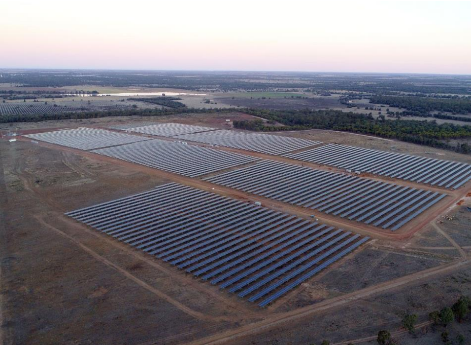
Solarpark Chincilla in Queensland
