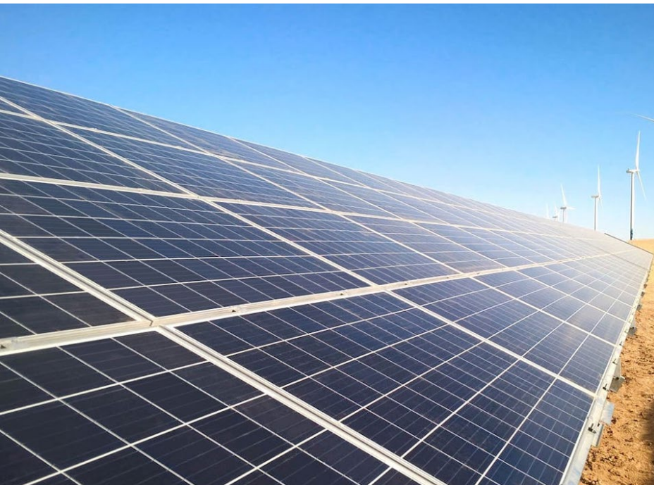
Solarpark Sainshand, Mongolei
